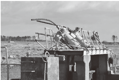
In Yuriage, huge wave destroyed water gate.
